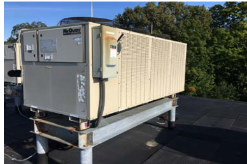
Batchelder Rooftop Unit
