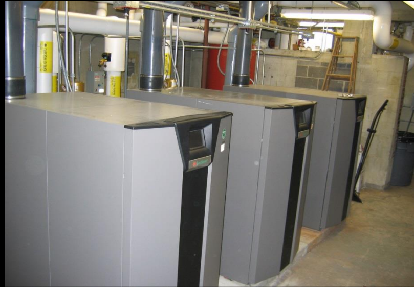
Little School Boilers
