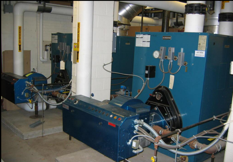
Hood School Boilers
